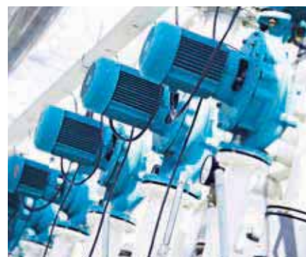
Water Supply & Water Treatment
