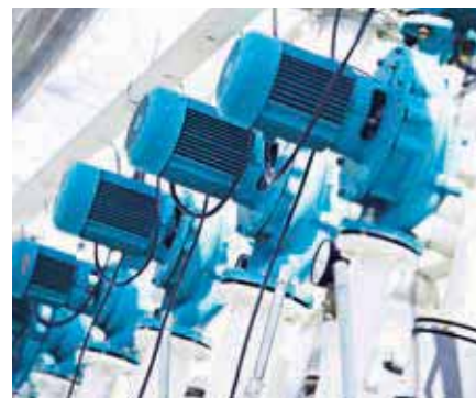
Water Supply & Water Treatment
